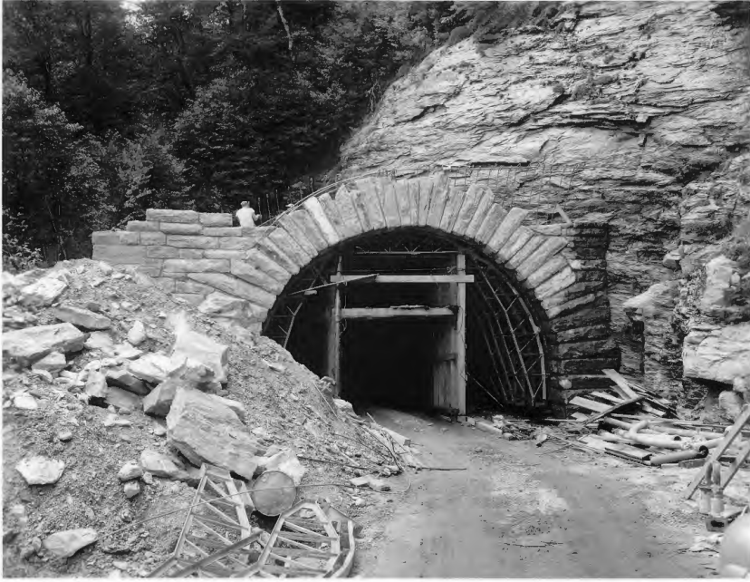
The Blue Ridge Parkway under construction. The road and its surrounding scenery were constructed, but they were also meant to blend into each other. The tunnel portal under construction showcases the meeting points between human work and geological forces. National Archives, College Park, Maryland, Special Media Archives, Still Picture Unit, 55-1813
